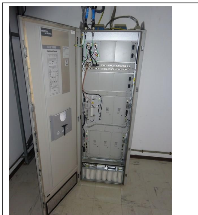
Figure 11 : Baie Nortel S1800 INDOOR GSM* 900
